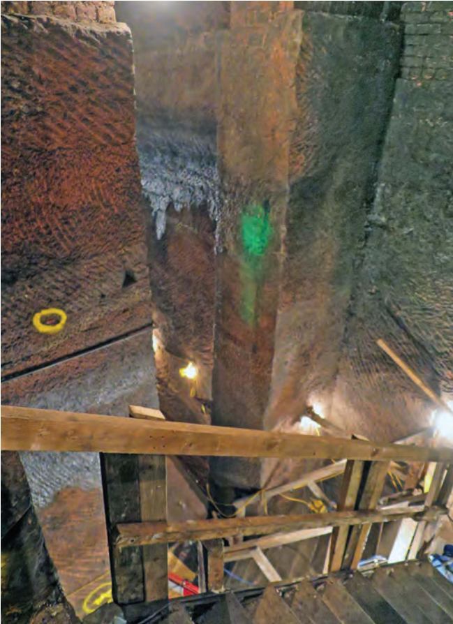
Hand carving marks on the sandstone walls of the reservoir chamber, with detailed brickwork above. Photo Clive Penfold
